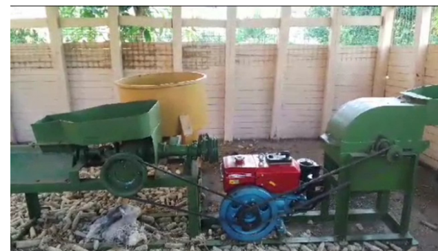
Installed motorized briquette machine in Kyabatalya Community Efficient cook stove Making & Briquettes for business in Kikube district
